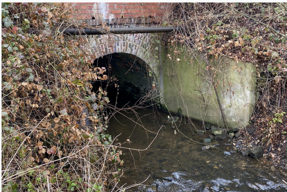
Not here, please. A beaver has tried to settle on this railway embankment in the Jülich Börde.
